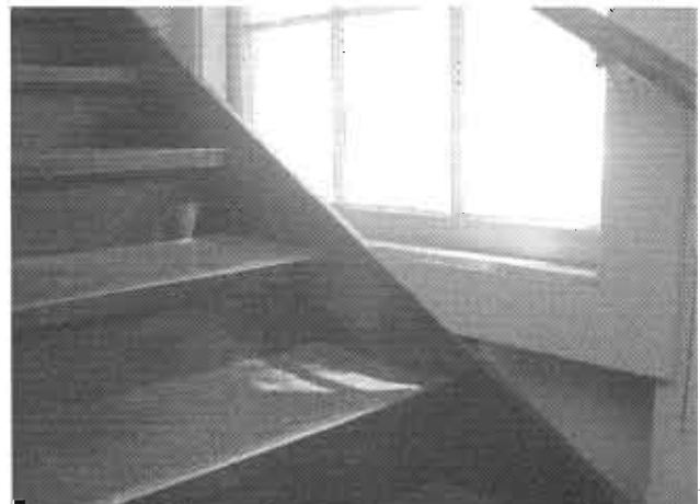
Figure 25. Relocated stair stringer crosses windows
