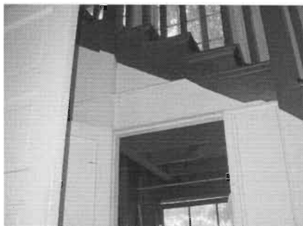
Figure 30. Altered stair landing at Room #208
