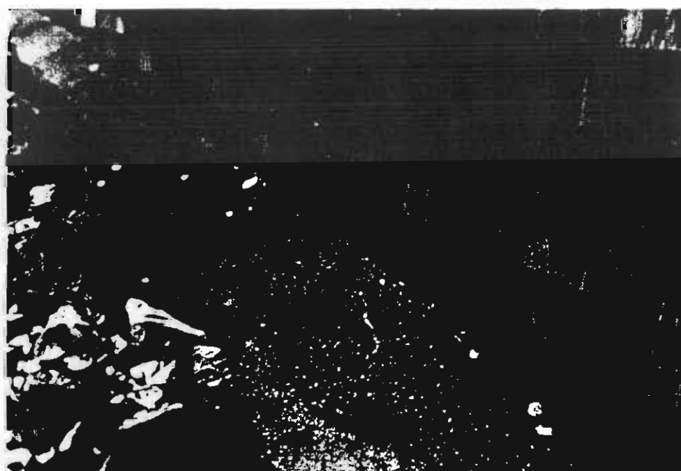
1b. Sill at grade conditions: Black top at sill near center of north elevation.
